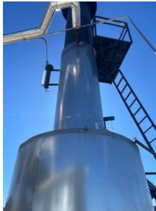
Biomass boiler + Particle filter
